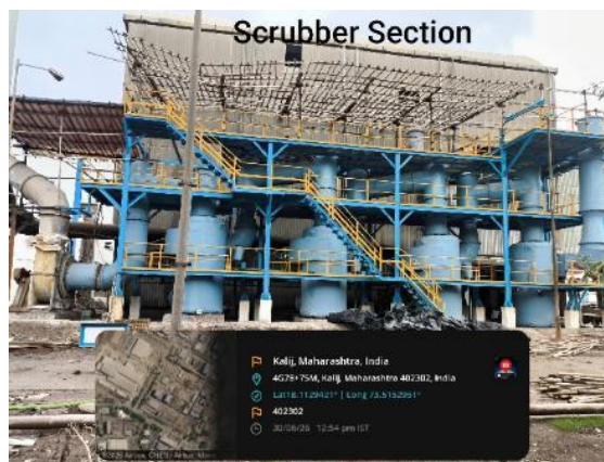
Scrubber – Mahad facility
