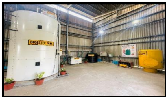
Bio digester plant – Goa facility
